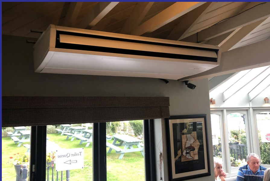
New air conditioning system installed by CS HVAC at The Halfway House Restaurant
